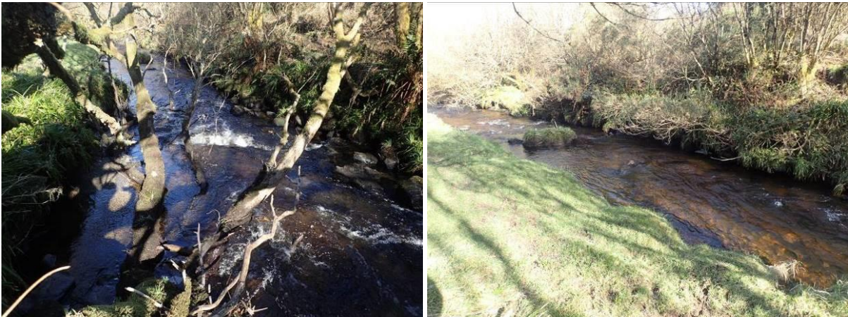
Plate 21 Build up a large secure notch weir at primary riffle to yield a high drop into plunge pool. Cut willow at riffle. View upstream (left) view from instream (right).
