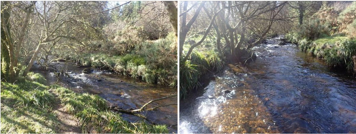
Plate 20 Installation of a notch weir by adding to the existing boulders at existing riffle. View upstream (left), view from instream (right).
