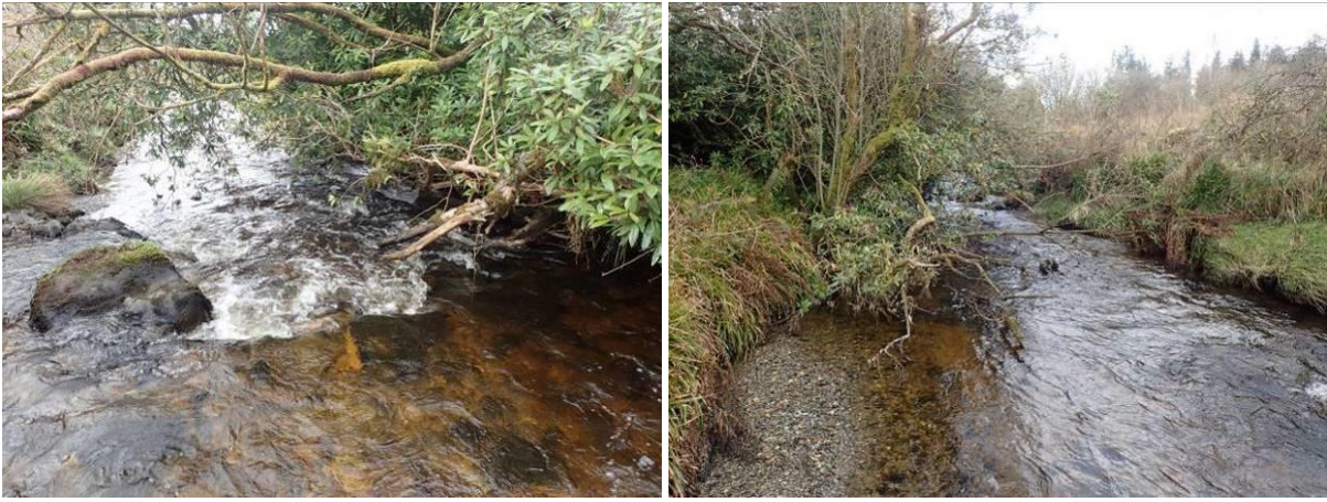
Plate 4 Location 4 Installation of notch stone weir and removal of Rhodendron. Downstream view (left) and upstream view (right).
