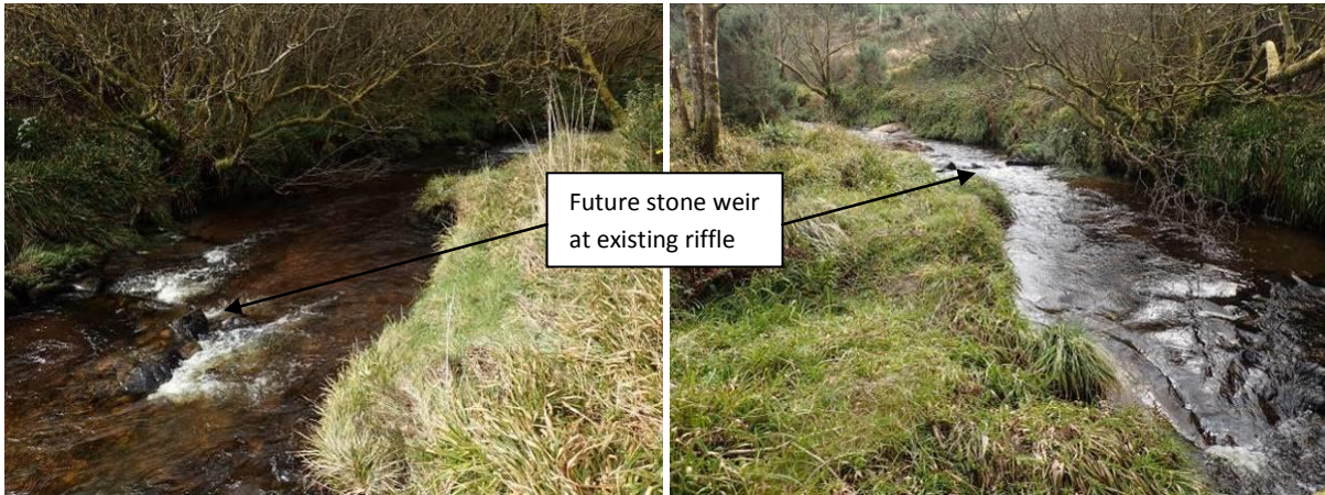
Plate 6 notch stone weir to direct flow to right away from eroding left bank. View downstream (left) view upstream (right).
