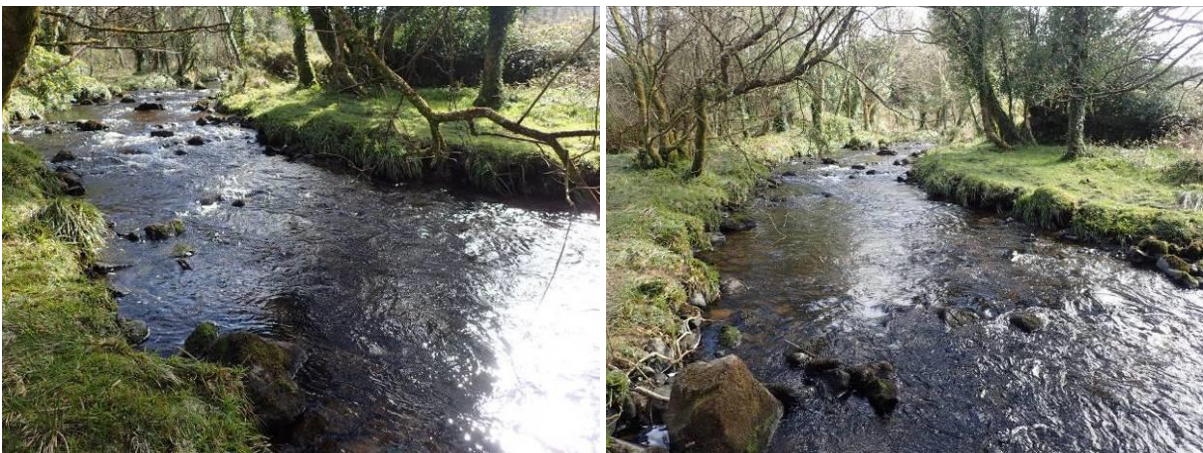
Plate 39 Move instream boulders to primary riffle to direct flow to center. Clear lateral branch.
