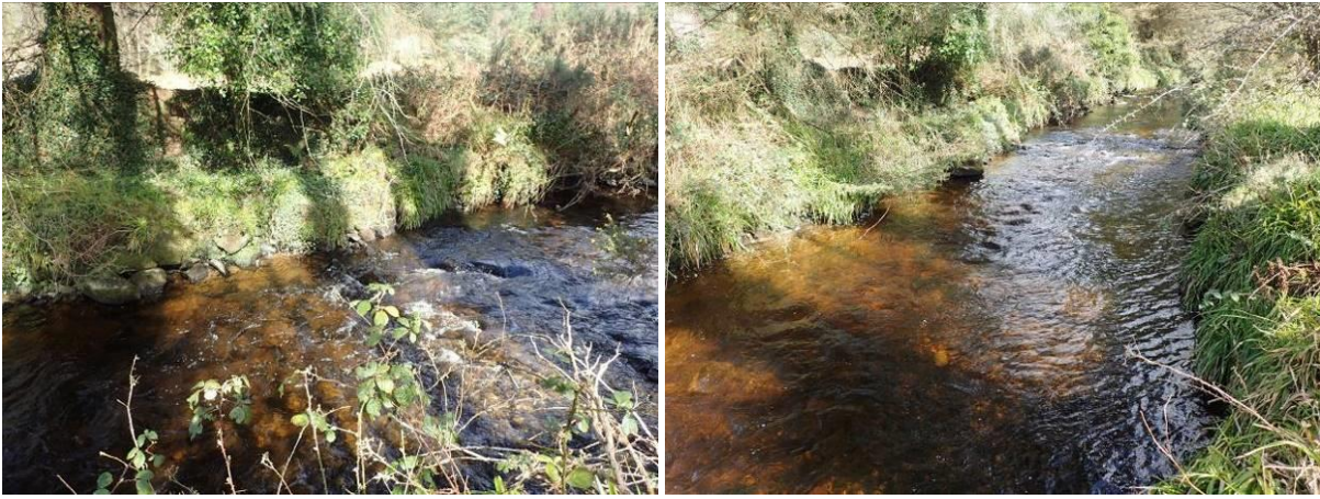
Plate 37 Create notch weir at narrowest part of stream ca. 4m upstream of large Sitka spruce tree (left). Upstream view (right).
