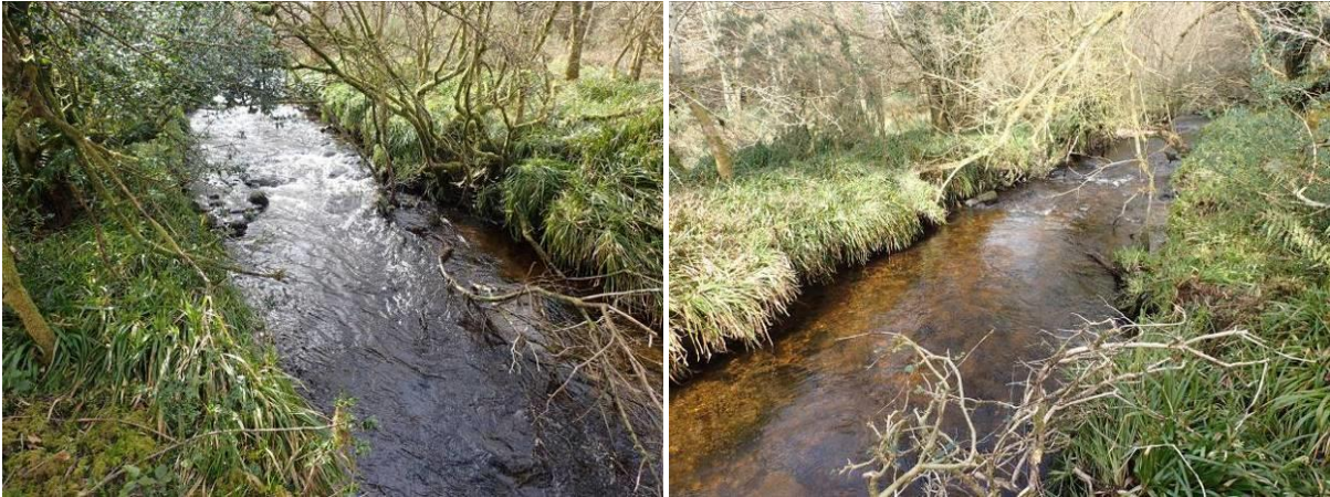
Plate 17 Installation of a notch weir by adding to the existing boulders at existing riffle. View upstream (left) view downstream (right).
