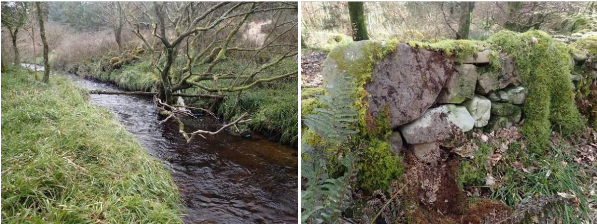
Plate 14 Undercut banks here would benefit from hydrodynamic alteration: redirecting thalweg to the centre of channel (left). Bank reprofiling also recommended. Source of stone nearby (right).
