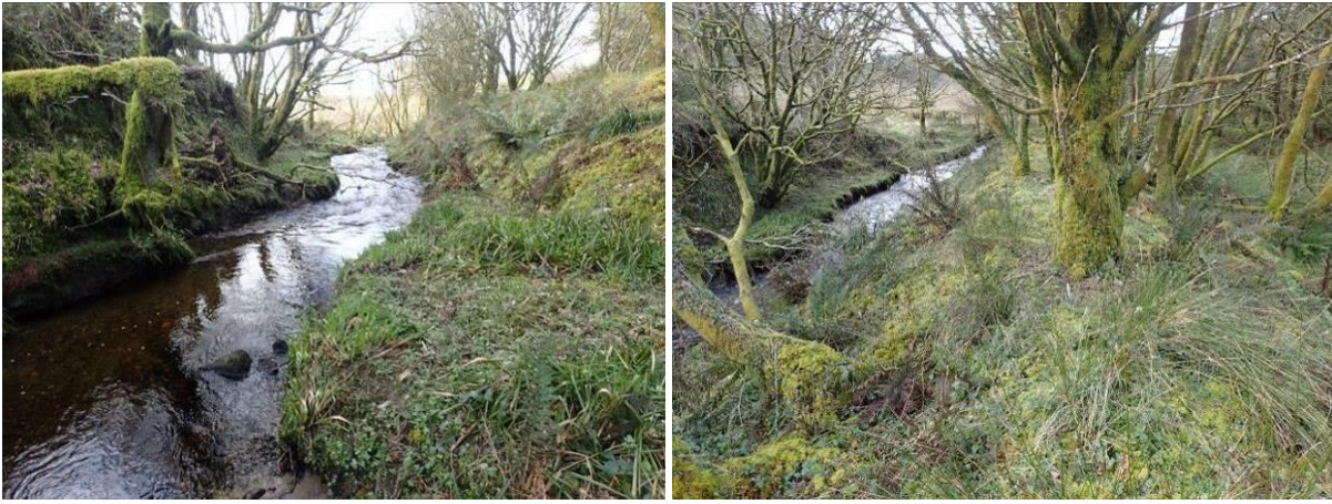
Plate 1 Location 1 on the Coumnagun Stream: placement of random boulders instream and stone weir (left).
