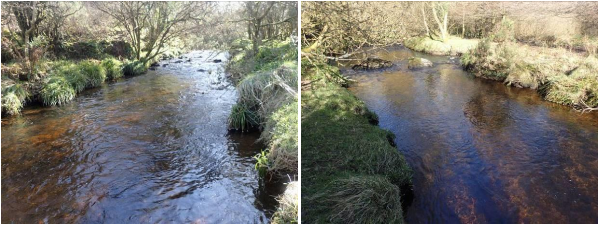
Plate 19 Installation of a notch weir by adding to the existing boulders at existing riffle. View upstream (left), view downstream (right).
