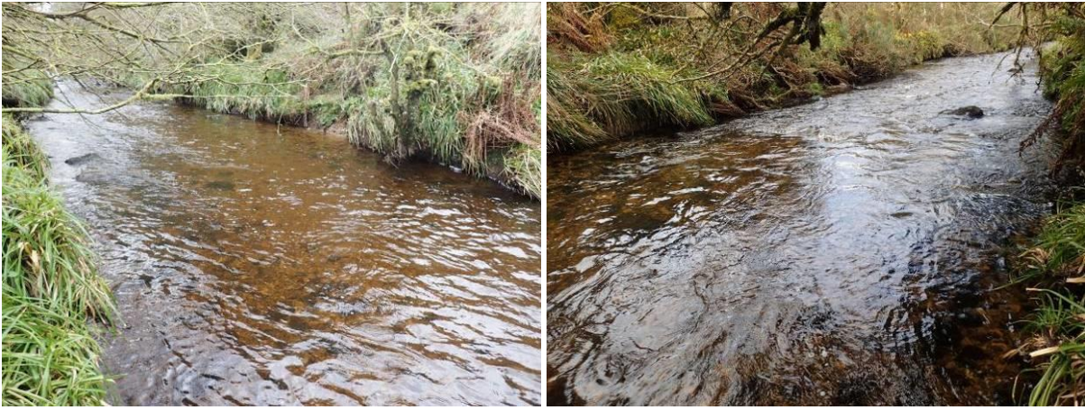
Plate 16 Installation of a notch weir, with pool head at existing riffle. View upstream (left) view downstream (right).
