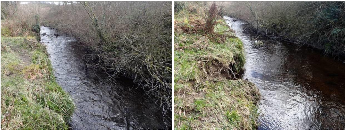
Plate 38 Move instream boulders downstream to main riffle to create a notch weir (left, background). Grade RHS bank and protect as it is undercutting, and protect with rock armour/logs, as available.
